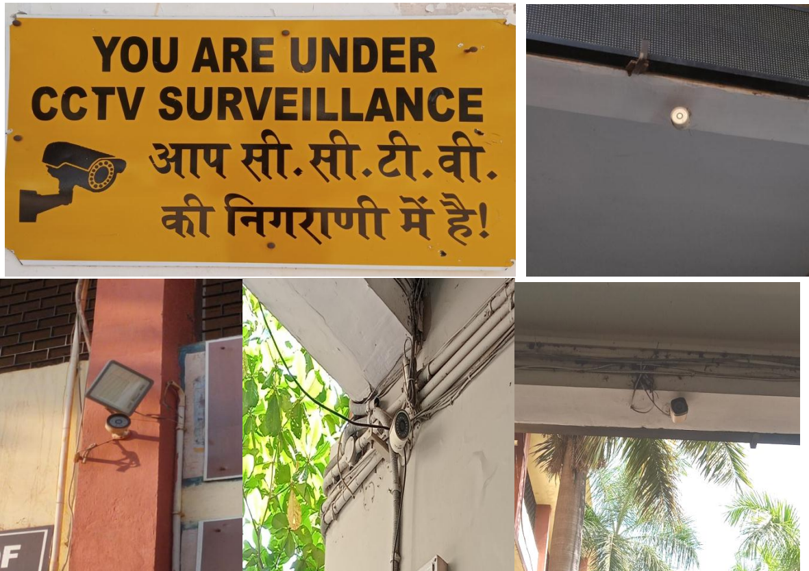
CCTV Cameras Installed in College Campus
